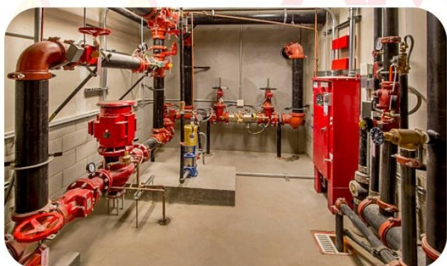
Fire Pumps + Panel
